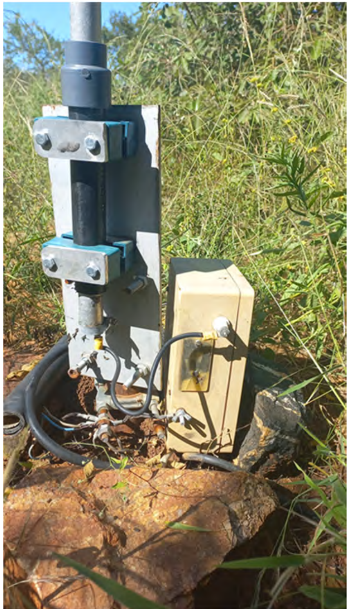
Fig. 2. Antenna base showing clamps, mounting plate and weatherproof box containing the matching circuits and relays.
