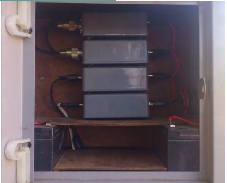
The Antenna Switch, the ZS0BOT beacon, the Cell Controller, the Solar Regulator/charger, two 7 A/h Battery packs and the GSM module
