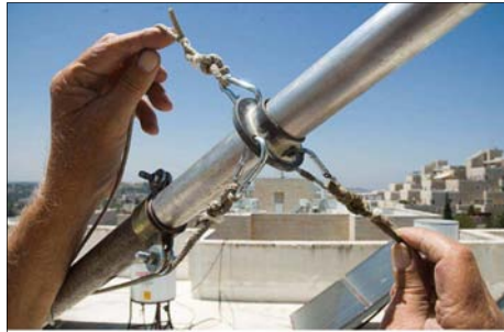
Picture 3: The omega clamps and a flange at 4X4LH's roof
